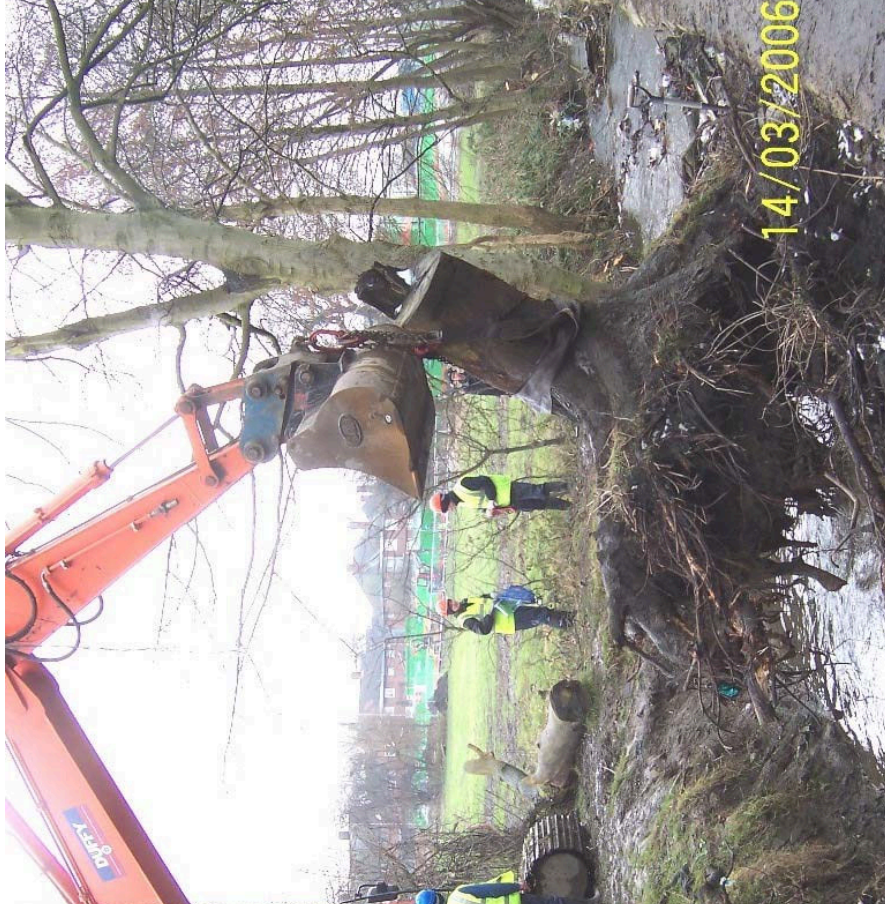
Removal of a mature tree from the centre of Wyke Beck (behind the Foxwoods) as part of the planned maintenance. Flooding in May 2005 affected properties adjacent to this stretch of beck
